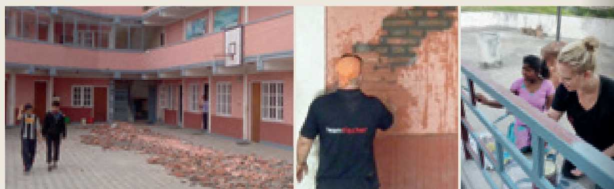
The damage caused by the earthquake could be repaired in the meantime
